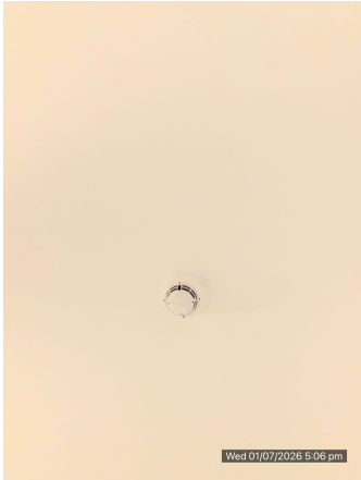
Security/Safety: Smoke alarms (photo 1 of 2)
